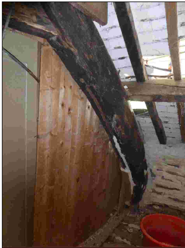
Plate 64: Slot in the northern blade of Truss 3
