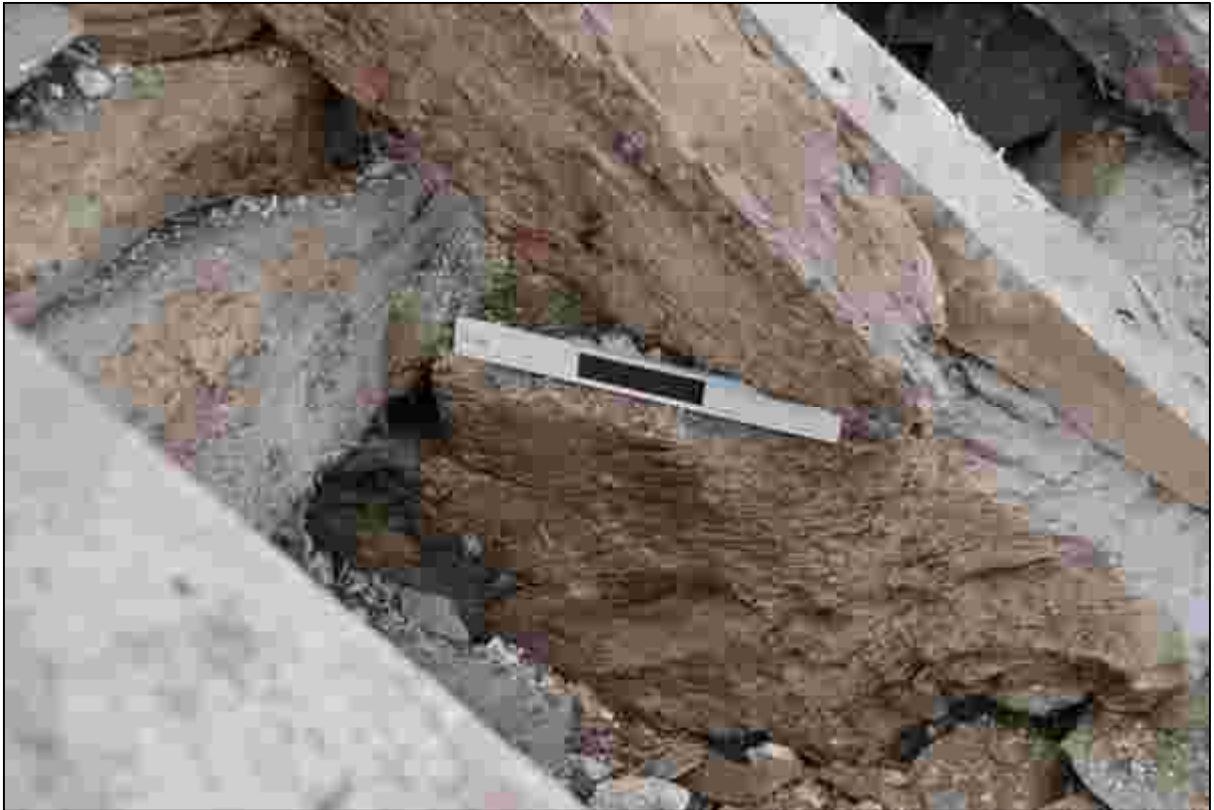
Plate 71: Spur between Truss 2 and the northern wall plate
