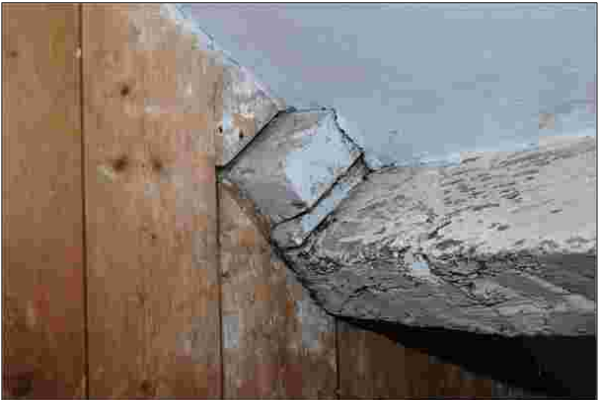
Plate 56: Overlap of the purlin in the eastern side of Bedroom 4
