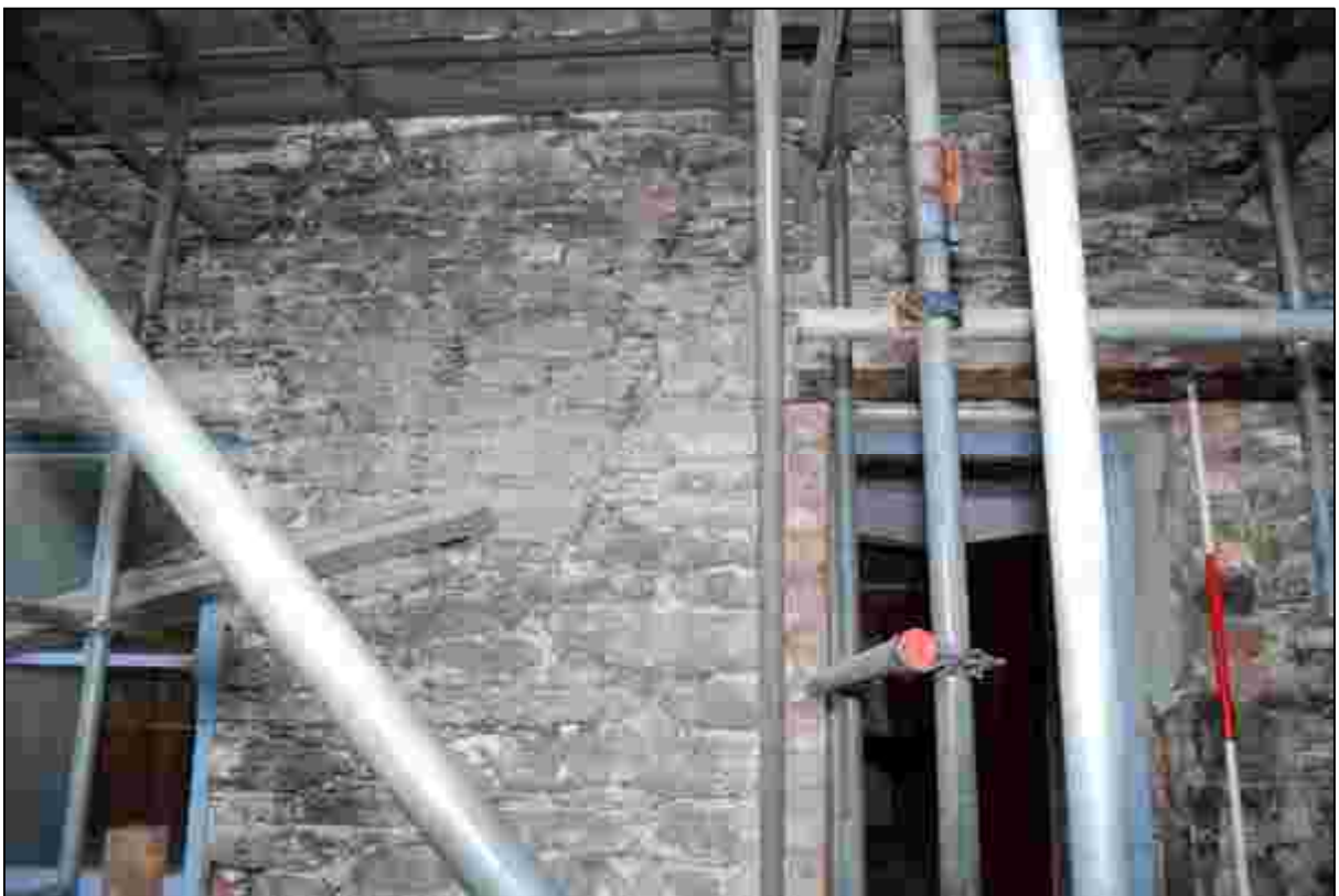
Plate 68: Crack in the stonework by the front door
