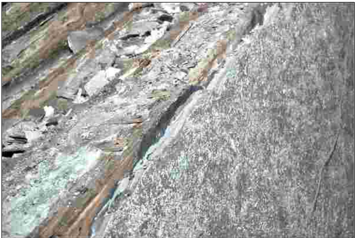
Plate 84: Chipping on the render of the western gable showing the slates below
