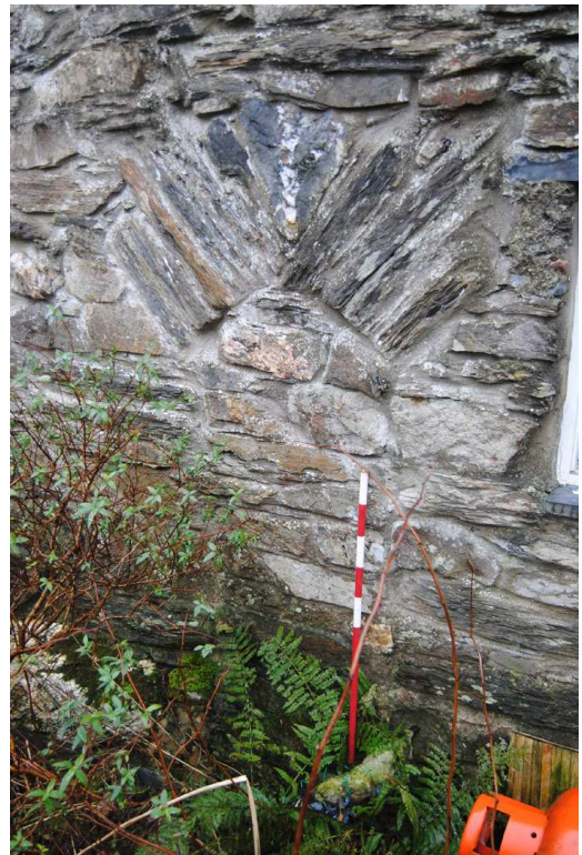
Plate 7: Blocked primary door to west elevation.
