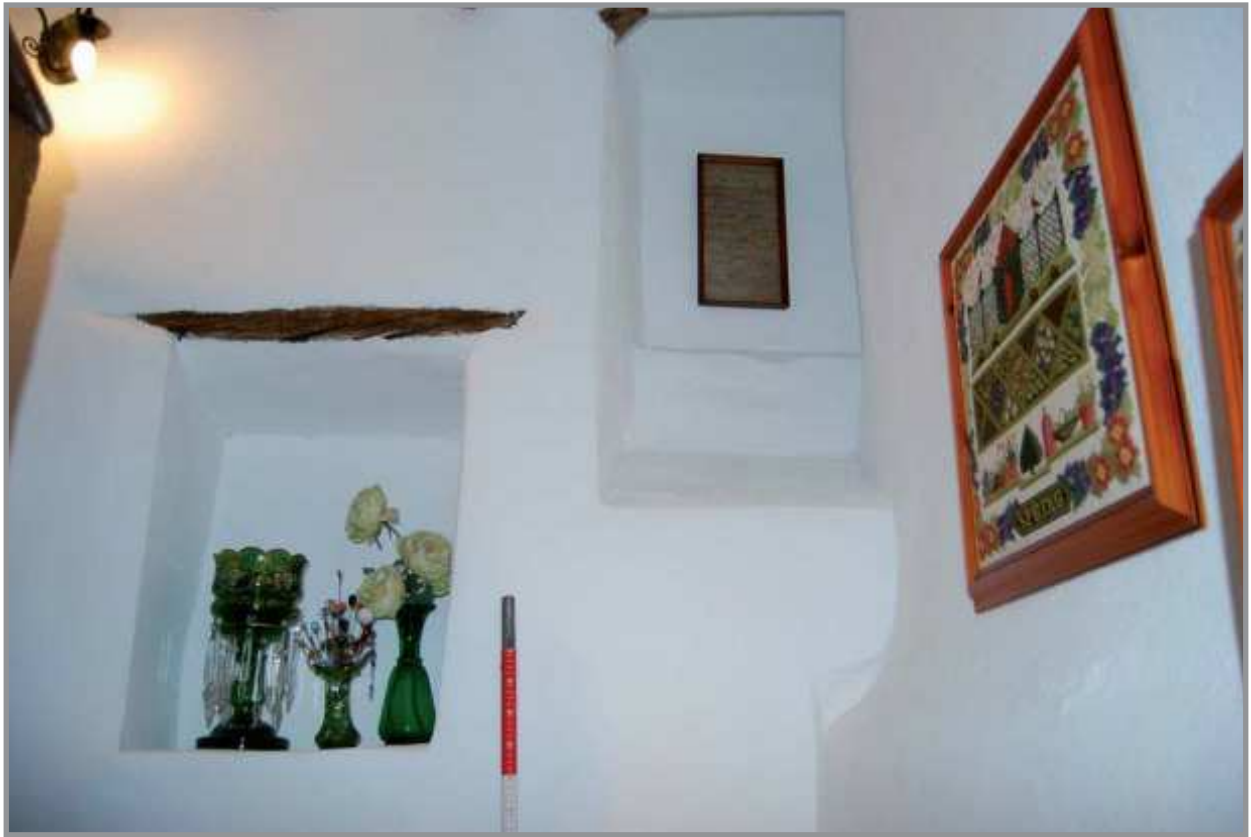
Plate 9: Stairway, showing blocked window. Facing south-west
